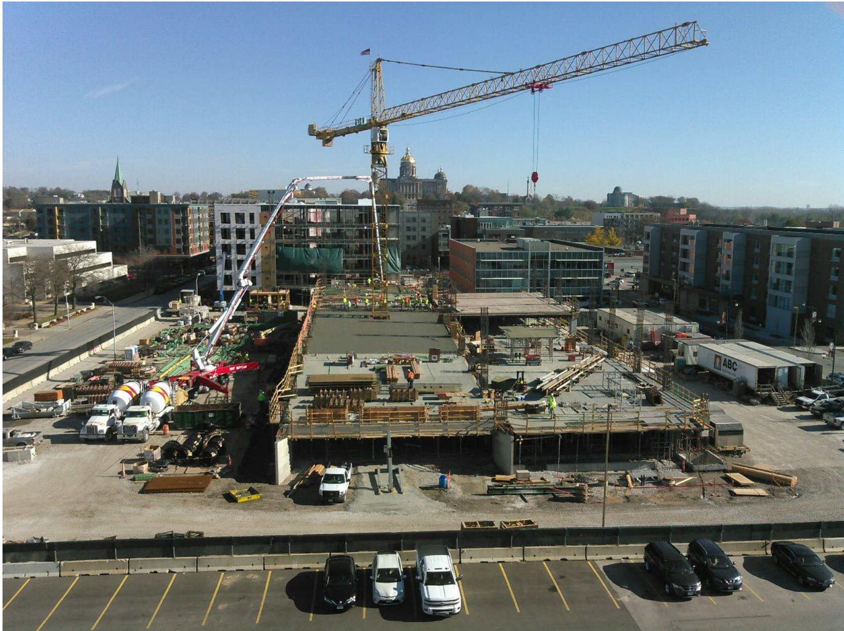
12/8/2016 - Work continues on constructing the elevated decks on the garage. The contractor is utilizing winter protection techniques to keep the construction moving forward.
