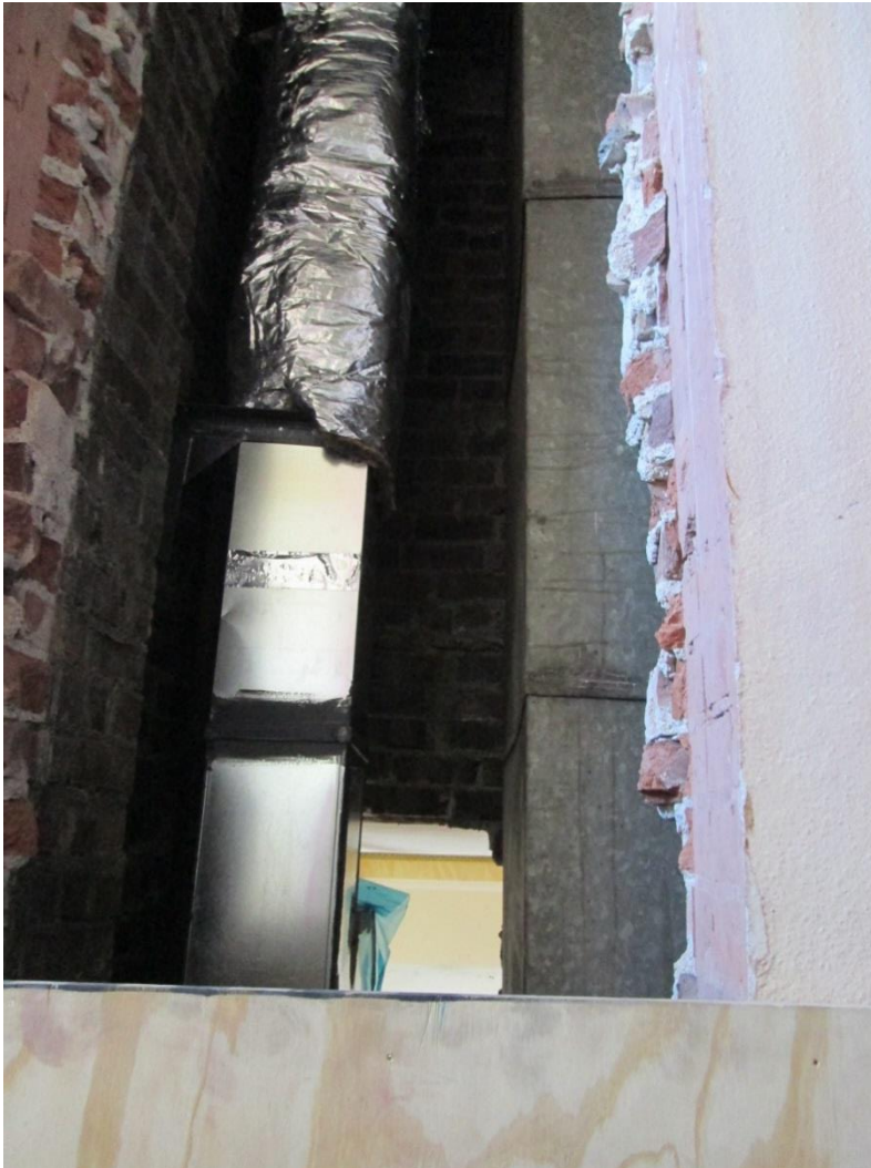
New insulated ductwork installed in shaft.
