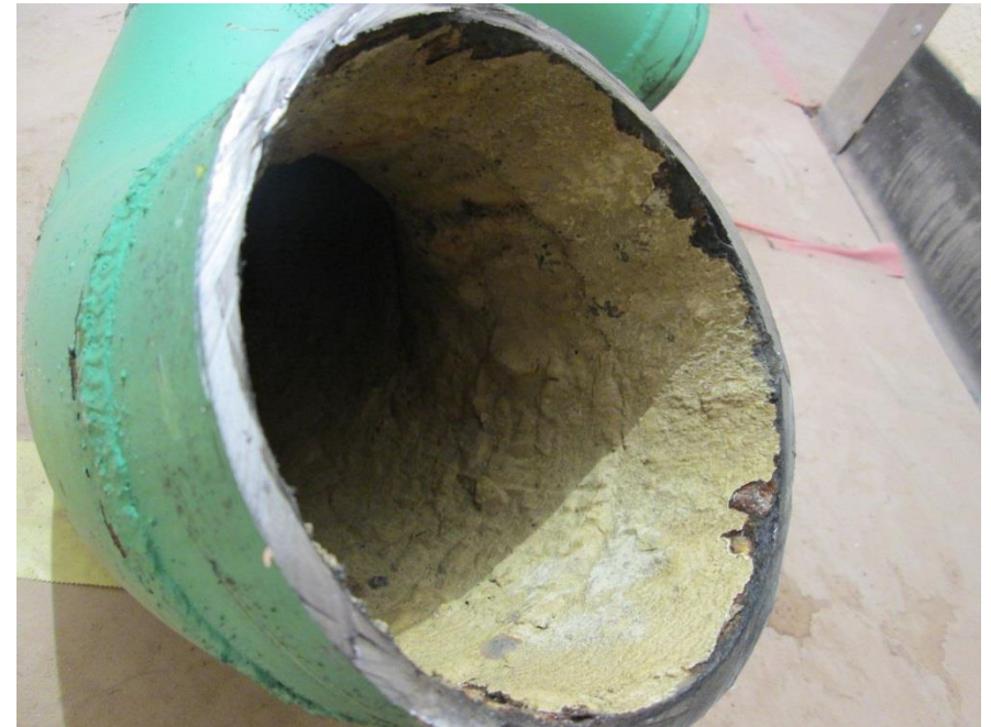
Existing pipe showing mineral build-up.
