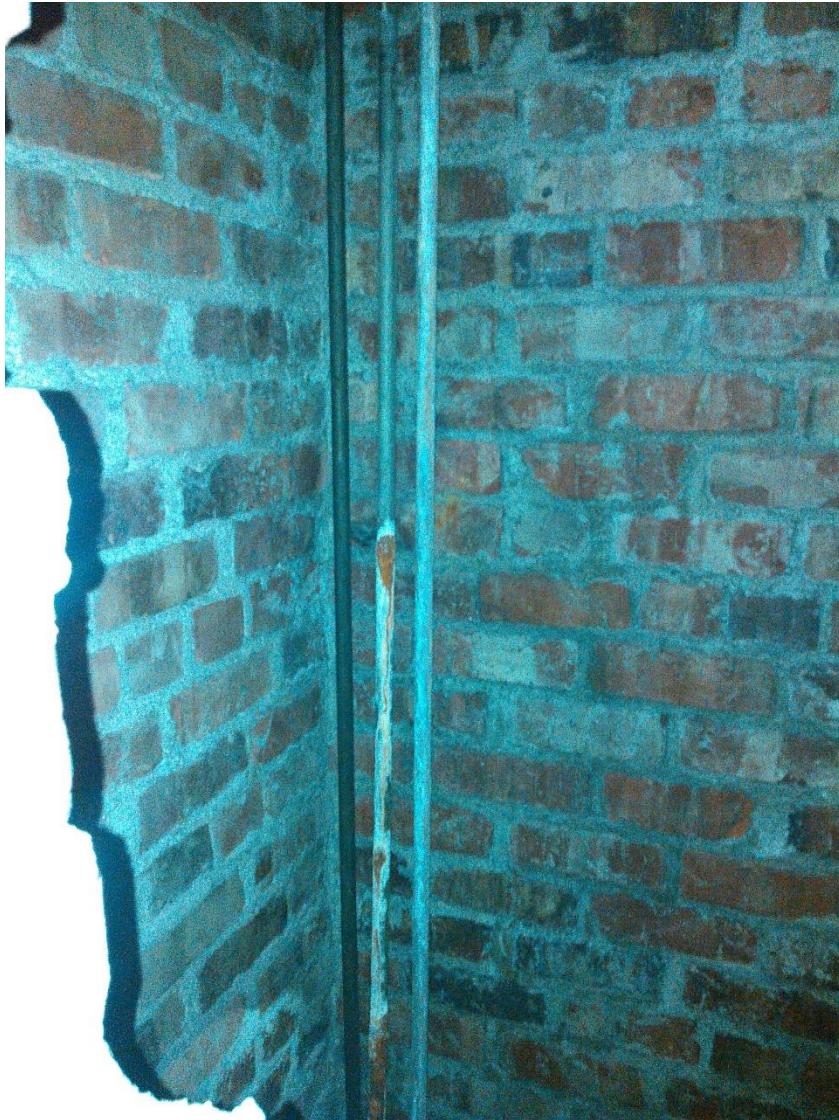
Deteriorated pipe in shaft.
