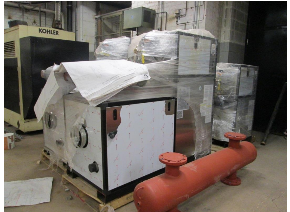
Three new boilers ready for installation.
