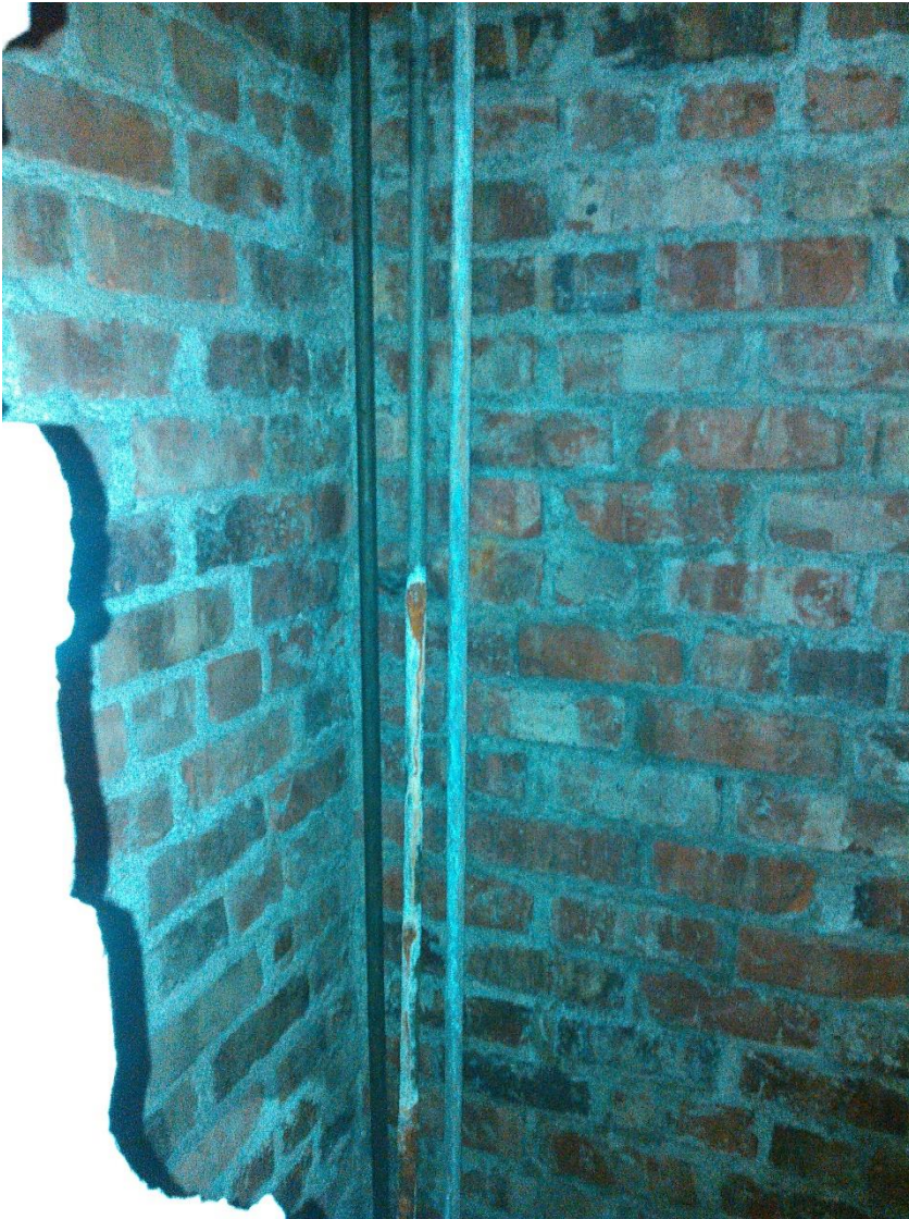
Deteriorated pipe in shaft.
