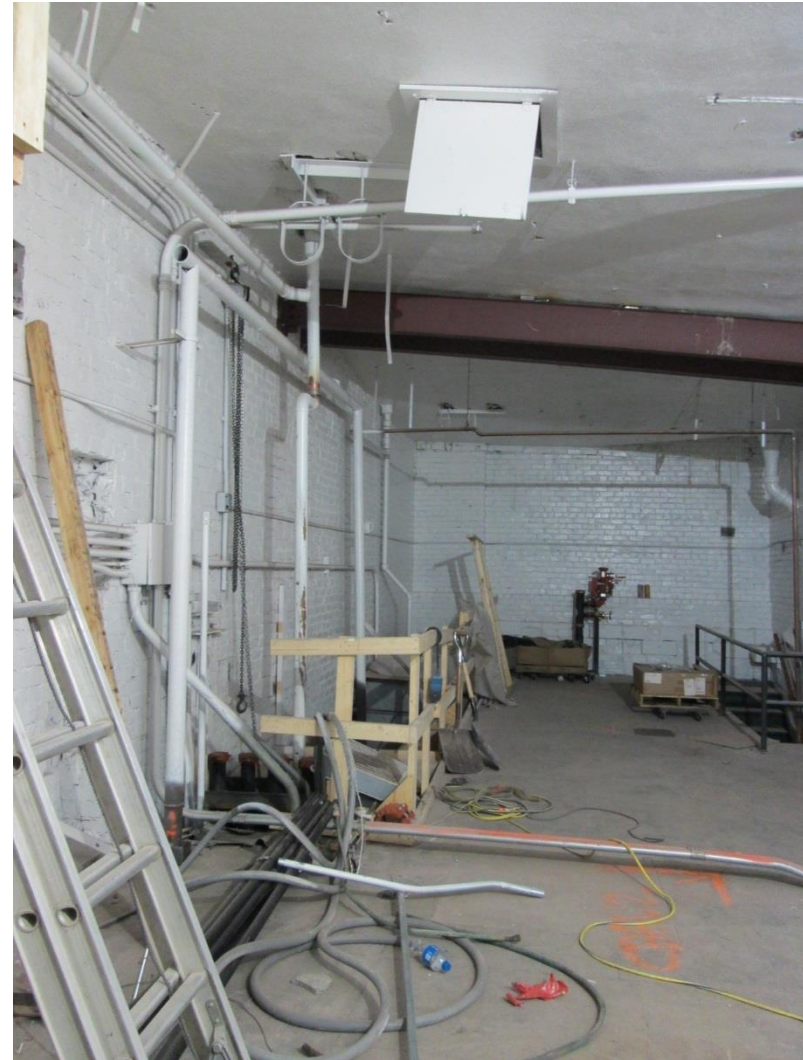
MECHANICAL ROOM IN ATTIC SOON TO BE FILLED WITH EQUIPMENT
