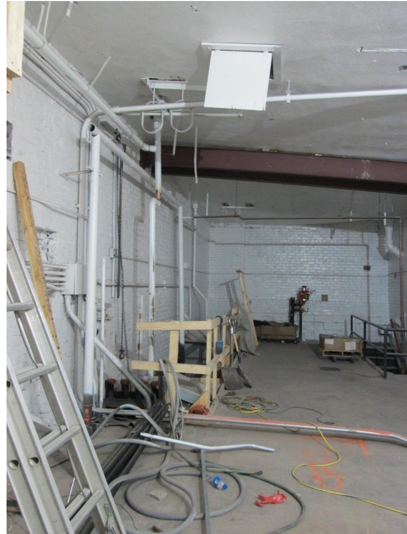
MECHANICAL ROOM IN ATTIC SOON TO BE FILLED WITH EQUIPMENT
