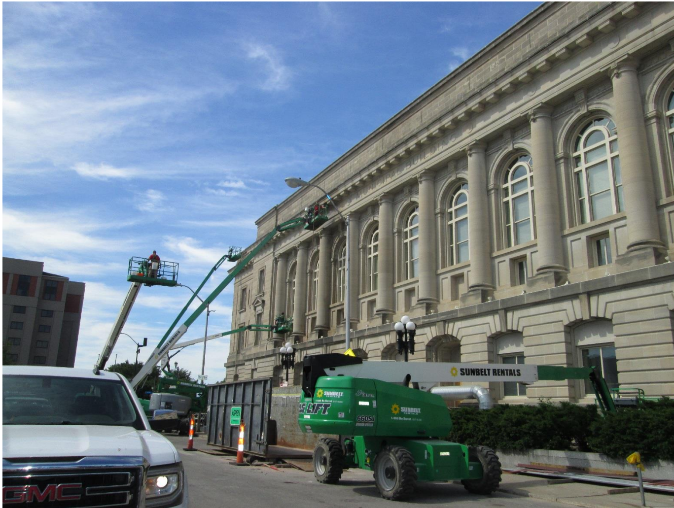
STONE REPAIRS AND TUCK POINTING UNDERWAY ON THE EAST SIDE OF CITY HALL
